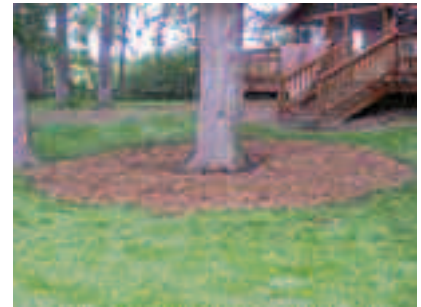
The finished treatment. This oak tree's roots are now in an improved environment and will benefit from the increased aeration and biological activity for years to come.
